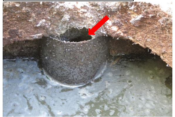
No effluent filter at outlet
